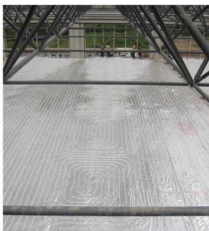
Fig. 8 – Underfloor heating made from Hostalen 4731 B – courtesy of Kingbull
