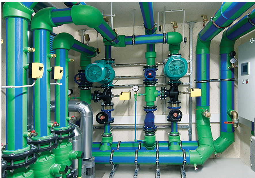
Fig. 10 – Heating distribution system made from PP-R – courtesy of Aquatherm
